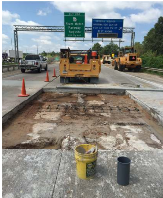
Figure 1. First Trial - Difficult Sub-soil Conditions and Inadequate Sub-surface Preparation.
