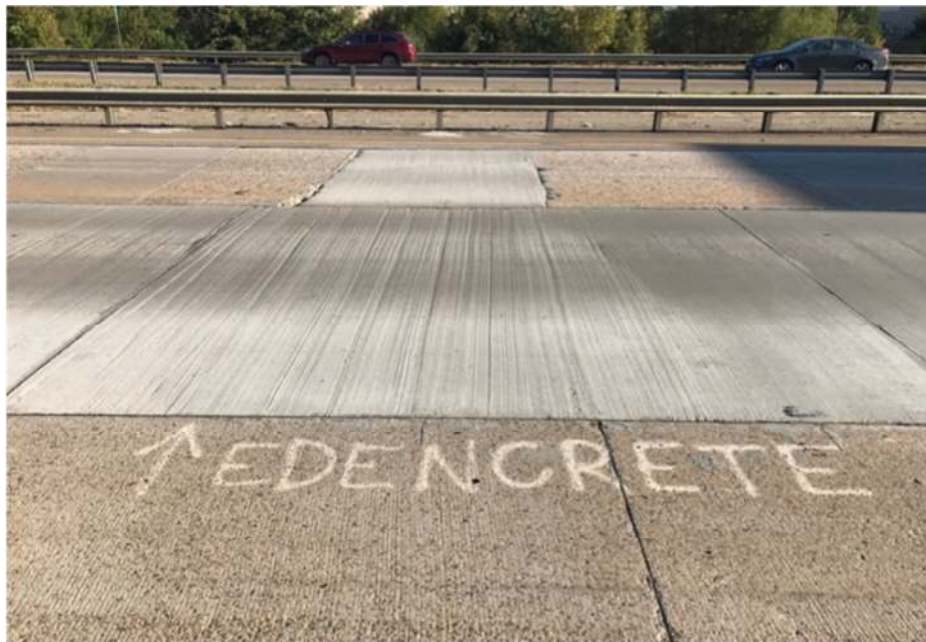
Figure 3. Second EdenCrete® Slab after 14 months (Oct 2016) - showing no cracking.
