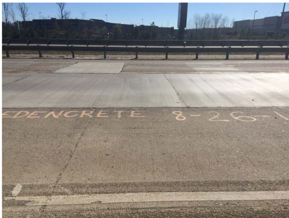
Figure 4 - Second EdenCrete® Slab after 18 months (19 Jan 2017) - showing a superficial crack.
