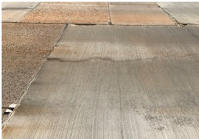
Figure 2. Second Reference Slab after 14 months (Oct 2016) - crack to full depth of slab.
